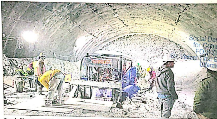
Nearly 50 metres of debris needs to be penetrated to insert the evacuation tubes.
